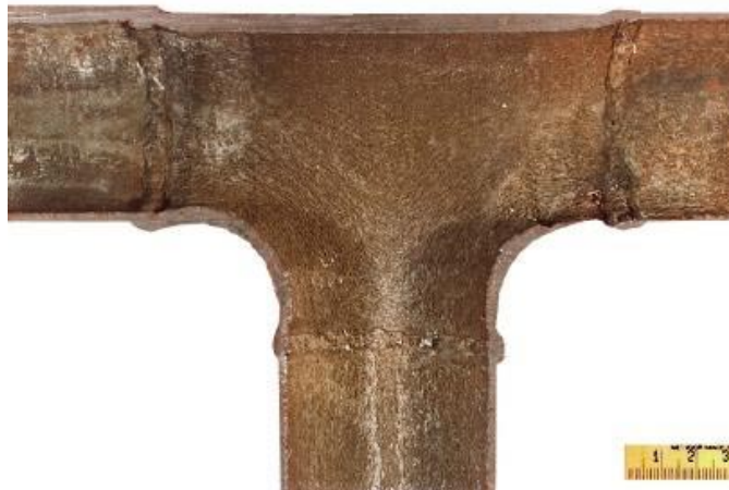
Figure 10: Erosion corrosion in a T-piece from a sulphuric acid line
