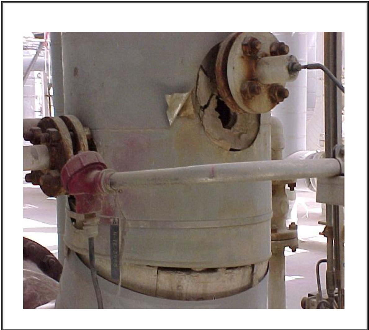
Figure 1 Missing Insulation Jacketing
