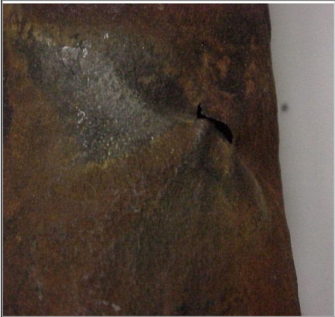
Figure 2 Failure of the 1.5 inch pipe due to CUI
